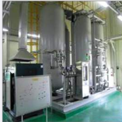
LG INNOTECH N 2 GENERATOR
