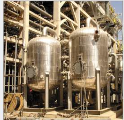
TUPRAS AIR DRYER
