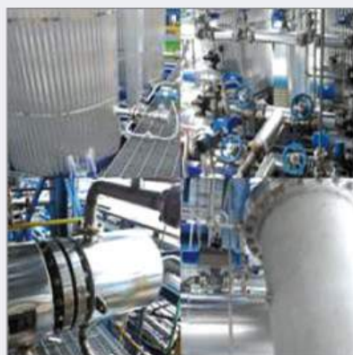
ISU CHEMICAL IPA DRYER
