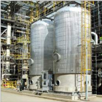
S-OIL N 2 RE-FINERY SYSTEM
