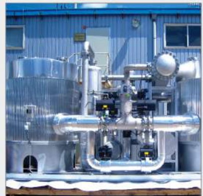
SK CHEMICAL N 2 DRYER
