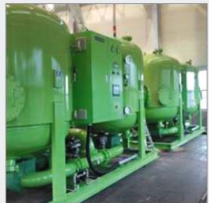
SAMSUNG TECHWIN AIR DRYER
